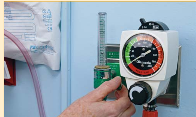
Figure 2. Adjusting flow rate.
